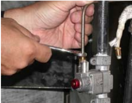
11. Carefully thread the brass fitting from the pilot gas line into the body and tighten using a 7/16" wrench.
