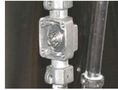
8. New spring/magnet assembly installed.
